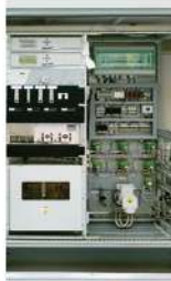
Continuous Emission Monitoring System
