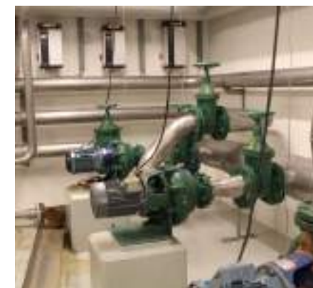
Marselisborg WWTP Motor Pumps
