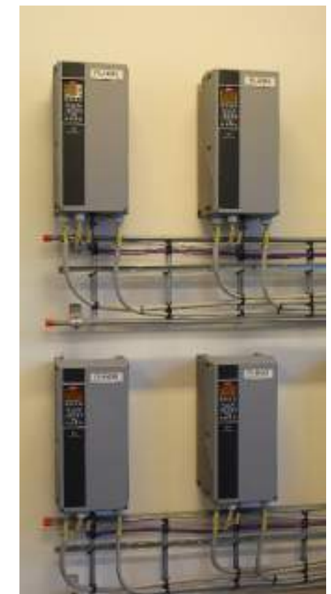
Marselisborg WWTP VLT Aqua Drive
